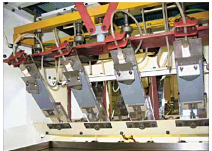
Surge Arrester silicone insulation testing
