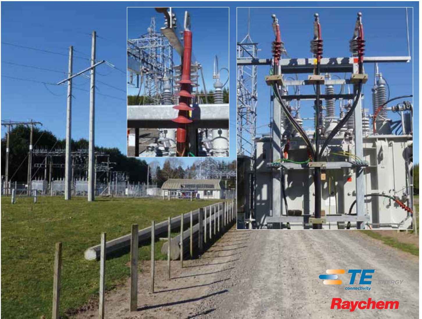
Te Matai Sub Station in the Bay of Plenty
